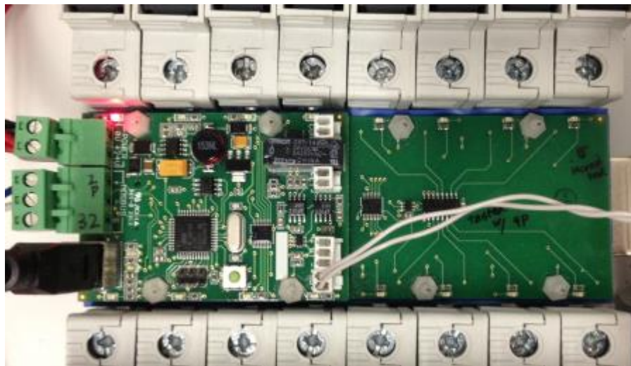
Figure 10. Channel 1 Light ON.
