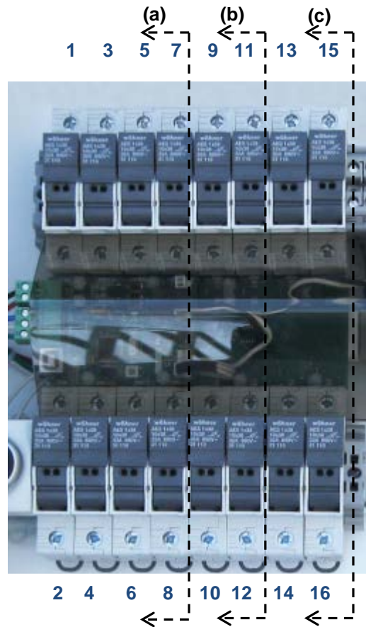
Figure 4. Input wire labeling schematic for (a) 8 strings, (b) 12 strings, and (c) 16 strings
