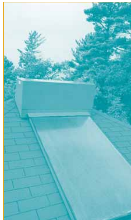
Thermosiphon solar water heater at Camp Queen Elizabeth, Beausoleil Island on Georgian Bay, Ontario. Courtesy of Solcan Ltd.
